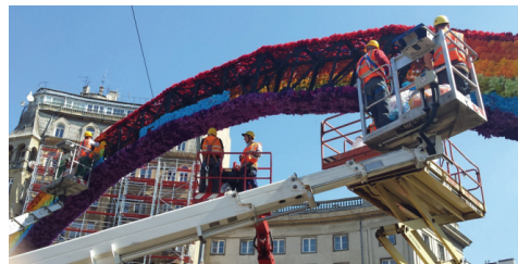
FIGURE 5. The process of the repair of 'Tęczą' after the fire (photo by T. Samsel, April 2014)
